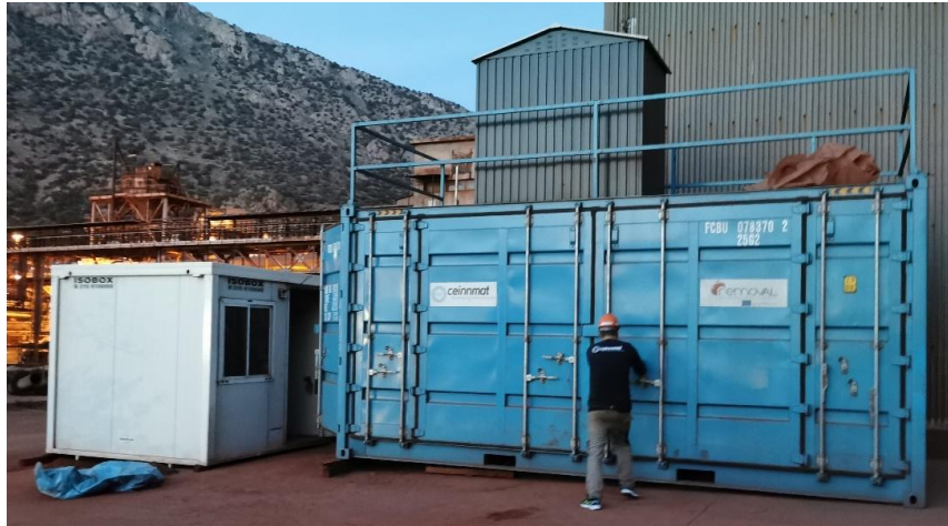
Figure 3. Installed Microwave Pilot Plant in MYTILINEOS.
